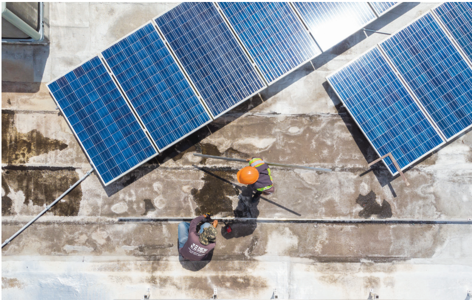
In Puerto Rico, AmeriCares installed solar energy systems to ensure health centers can function if future storms cut power.
